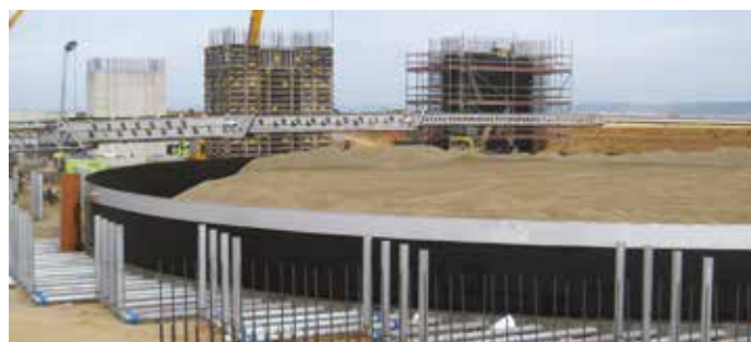
Merida Thermosolar Plant, Córdoba
